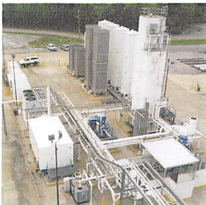
© UIG | UIG-owned and operated on-site for oxygen and nitrogen pipeline supply
